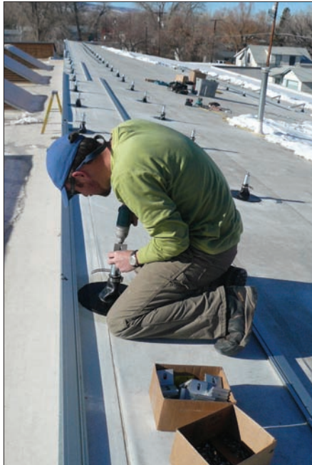
System engineer Phil Schneider affixes UniRac SolarMount standoffs to the roof in preparation for the installation.
