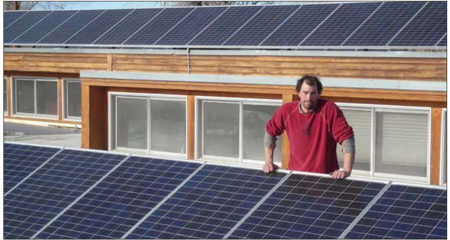
Creative Energies Electrician Josh Wells worked closely with local utility Rocky Mountain Power to ensure a smooth interconnection to the utility power line.
