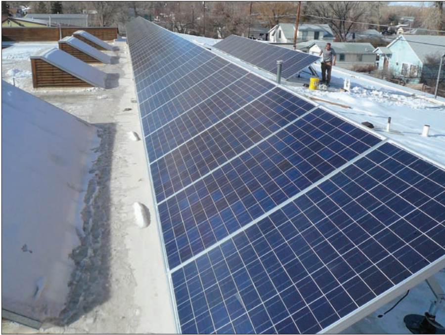
Though the school's maintenance crew must keep snow drifts from covering the modules, cold temperatures will not reduce output when the sun is shining.
