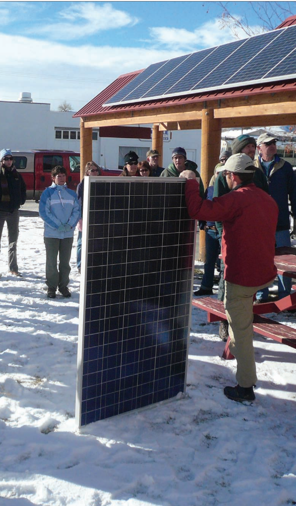
NOLS staff gets on-the-spot training from Creative Energies' Phil Schneider before pitching in to mount the solar panels.
